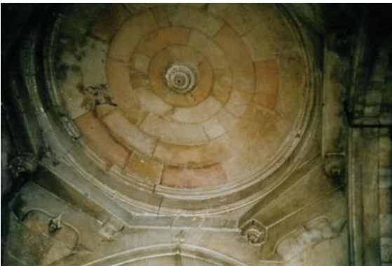
Building Construction. Fig. 12 Dome (Jumma Mosque, Ahmedabad). Ring forces balanced by overlapping; joints open where there is a little overlapping (photo by the author).
